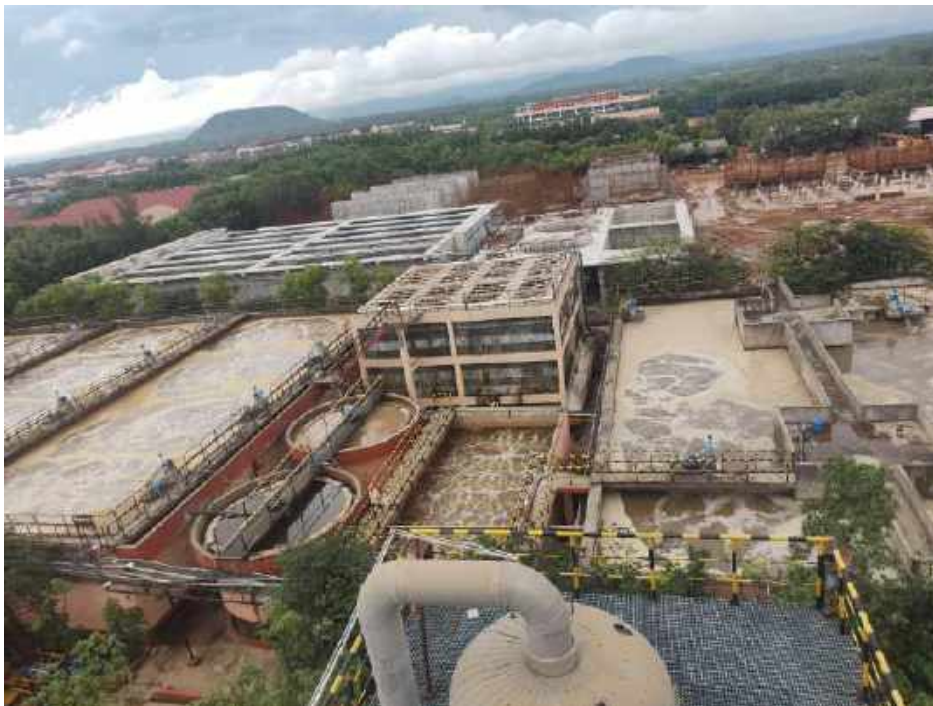
Fig. 1.9: Biological system for LTDS & Condensate of MEE & ATFD
